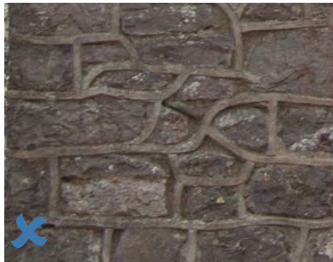
Inappropriate pointing to stone wall
