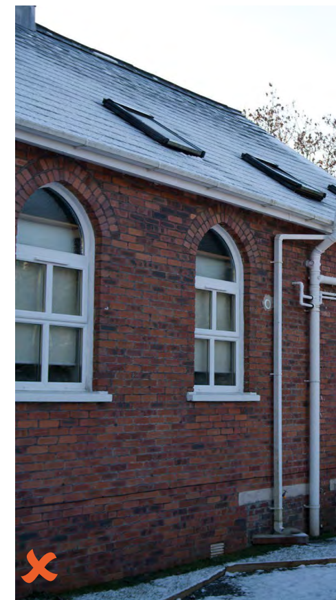
Above: external pipework and timber decking detract from the integrity of this residential chapel conversion
